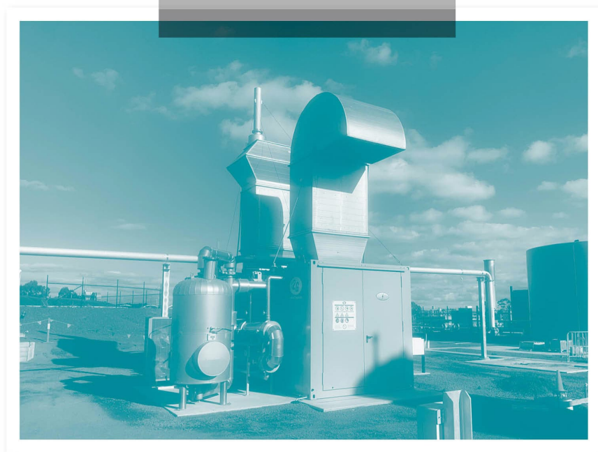
The new cogeneration unit powered by biogas at Colac Water Reclamation Plant.
